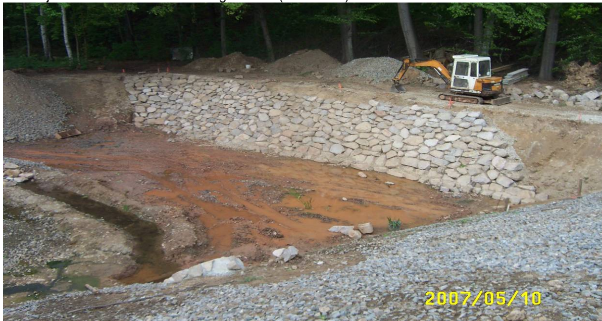
Sub-object 2: Rain retention basin Egersbach (fish ladder)
