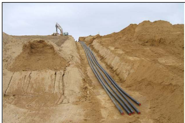
Track of the gas suction pipes
